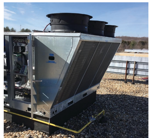
Installed Paragon HVAC at the Laboratory
