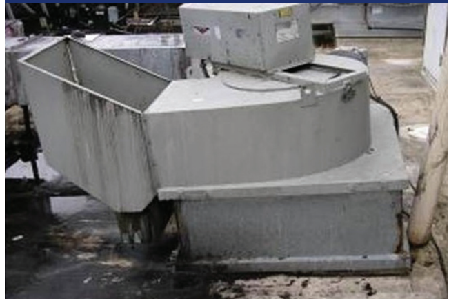
PHOTO 4 Exhaust Fan with Grease on Roof. Indicates how extensively grease can contaminate duct and fan system. Therefore best to keep them short, straight and vertical.
