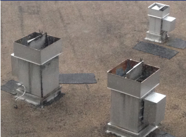
PHOTO 1 Grease exhaust fans with backdraft dampers locked in open position. Maintenance personnel got tired of dealing with dampers found stuck in the closed position.
