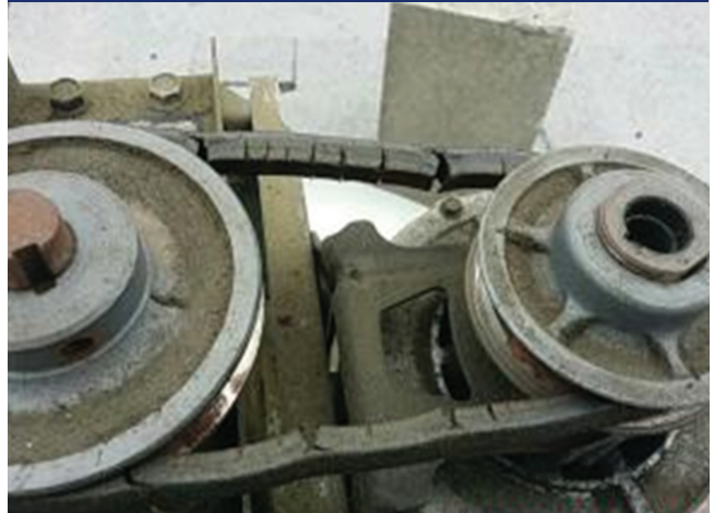
PHOTO 2 Stretched, cracked and almost broken belt. This is common for restaurant exhaust fans. Despite calls for proper maintenance by codes, this is often ignored.
