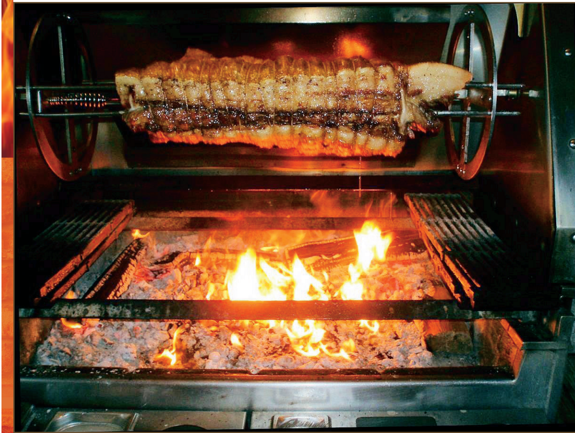
Figure 1. Commercial wood fired rotisserie and charbroiler (grates removed) above which fire ignited in the exhaust duct
