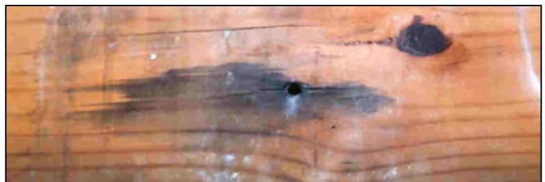
Figure 5. Heat damage on wood blocking.
