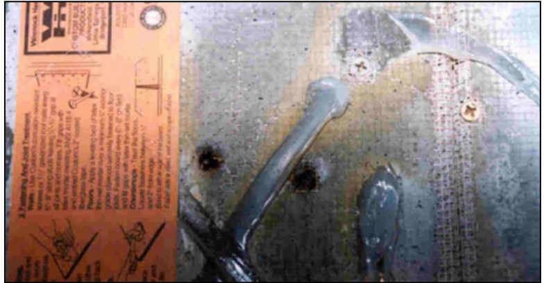
Figure 3. Heat damage on Durock® cementboard covering the wood blocking where the cheese melter hung
