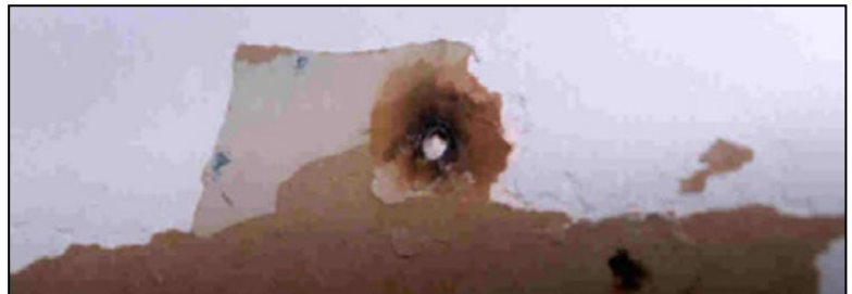
Figure 4. Heat damage on drywall covering the wood blocking where the cheese melter hung.
