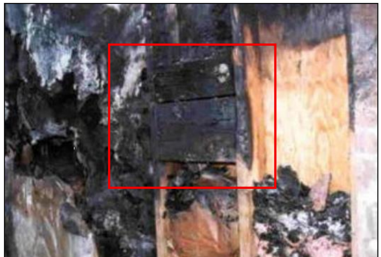
Figure 1. Origin area in the wall behind the cheese melter with the appliance removed.
