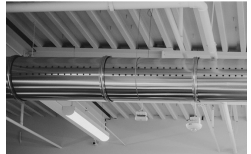
Figure 1 - CaptiveAire Supply Duct
