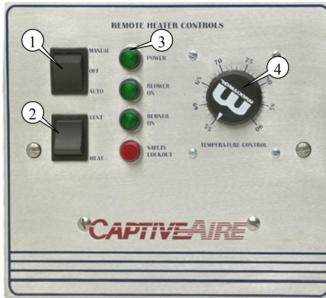
Direct Fired Remote Panel
